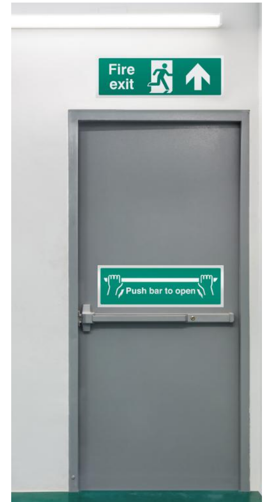
In compliance with EXIT SIGNS ON COMMON ESCAPE ROUTES 3.45 (Appendix 1)
